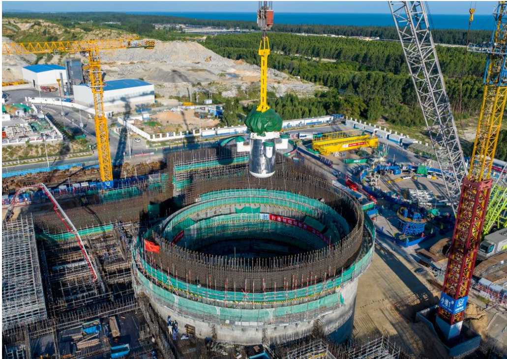
The core module of China's Linglong One, the world's first commercial small modular reactor (SMR), installed on August 10, 2023. (Photo: China News Service via Getty Images)
